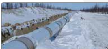
Completed Skin Trace system prior to burying
